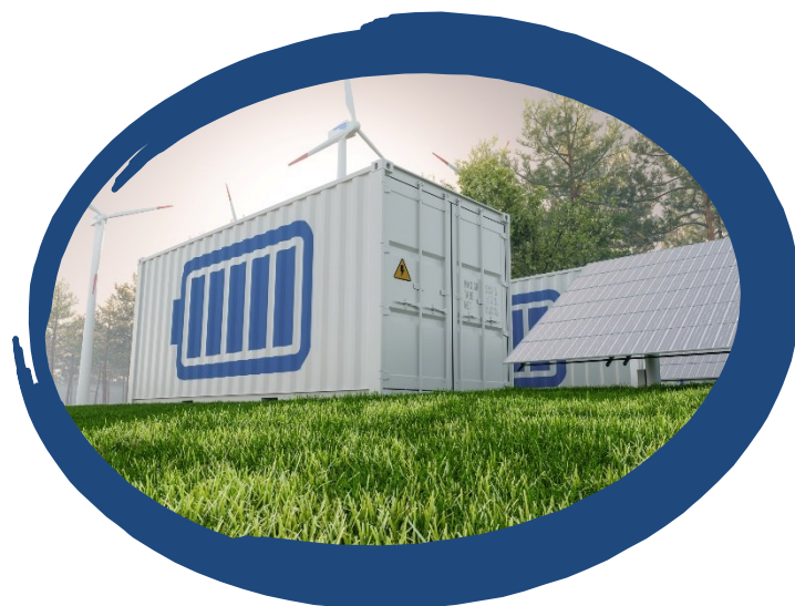
Figure 12: Battery Energy Storage System.
