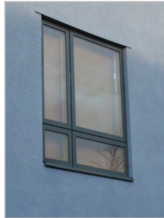
Position of glazing bars alters the character of the building
